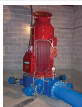
The District of West Vancouver is generating power from its drinking water system, with a 200 kW turbine that replaced a pressure-reducing valve.
