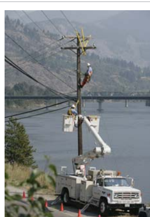
FortisBC crews working on a power line in Castlegar, next to the Columbia River.
